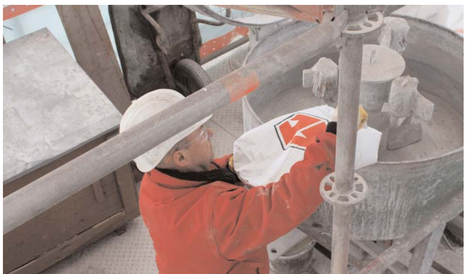
The SC-WearStop wear protection mortar is mixed up in a pan-pot mixer and manually applied by means of plastering trowel and finishing float. (Foto: wed)
