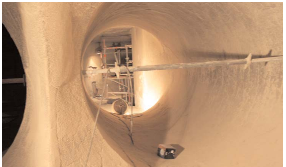
The riser dryer leading to the separator cyclones has a diameter of 2900 mm and is completely lined with SC-WearStop compound. (Foto: wed)
