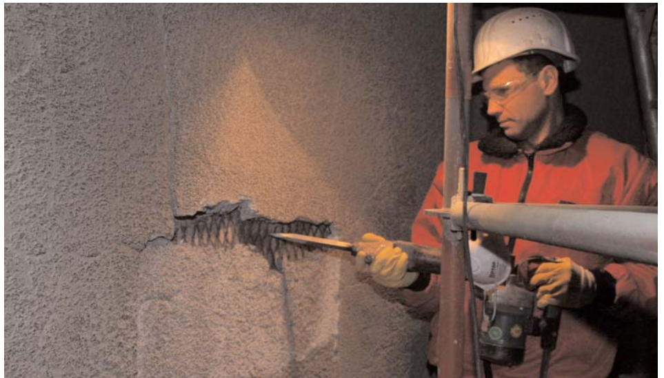
Individual and professional control and, if required, repair of the lining ensures a trouble-free production period for the operator (Foto: wed)
